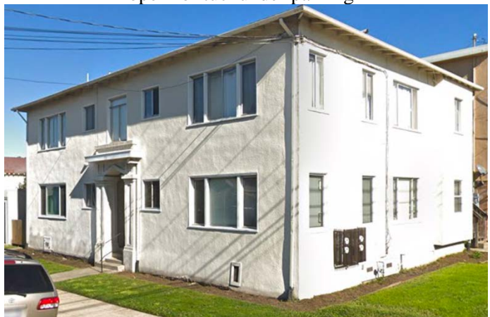
1f. 2-story, 4-unit. WFTS due to cripple wall
