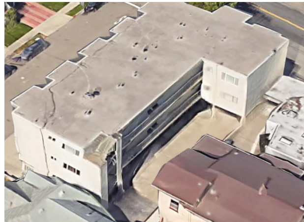
1d. 3-story, 12-unit. WFTS due to multiple wall lines open for tuckunder parking
