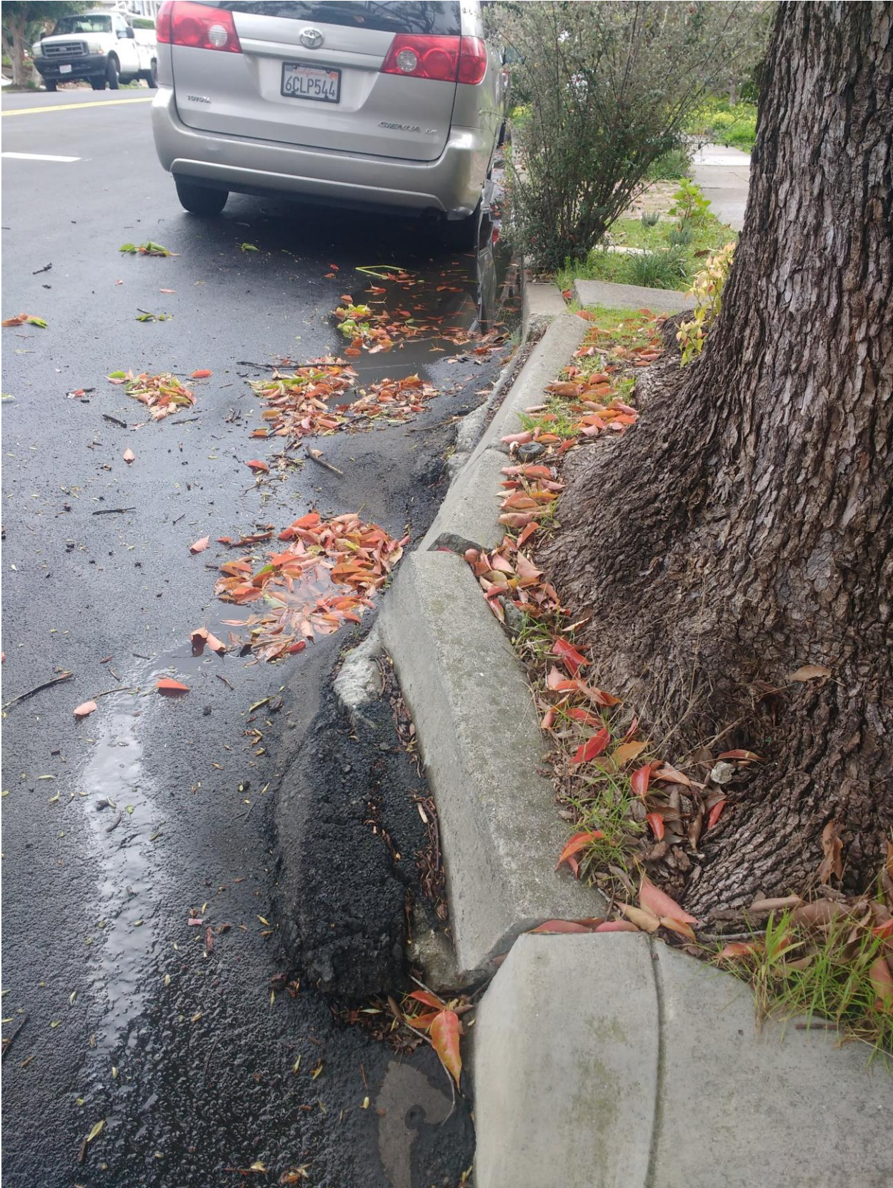
Damaged curb and gutter
