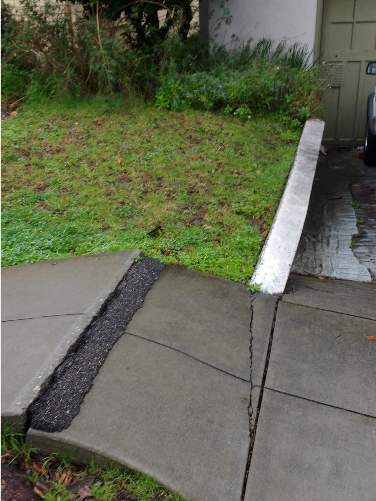
Pushed retaining wall
