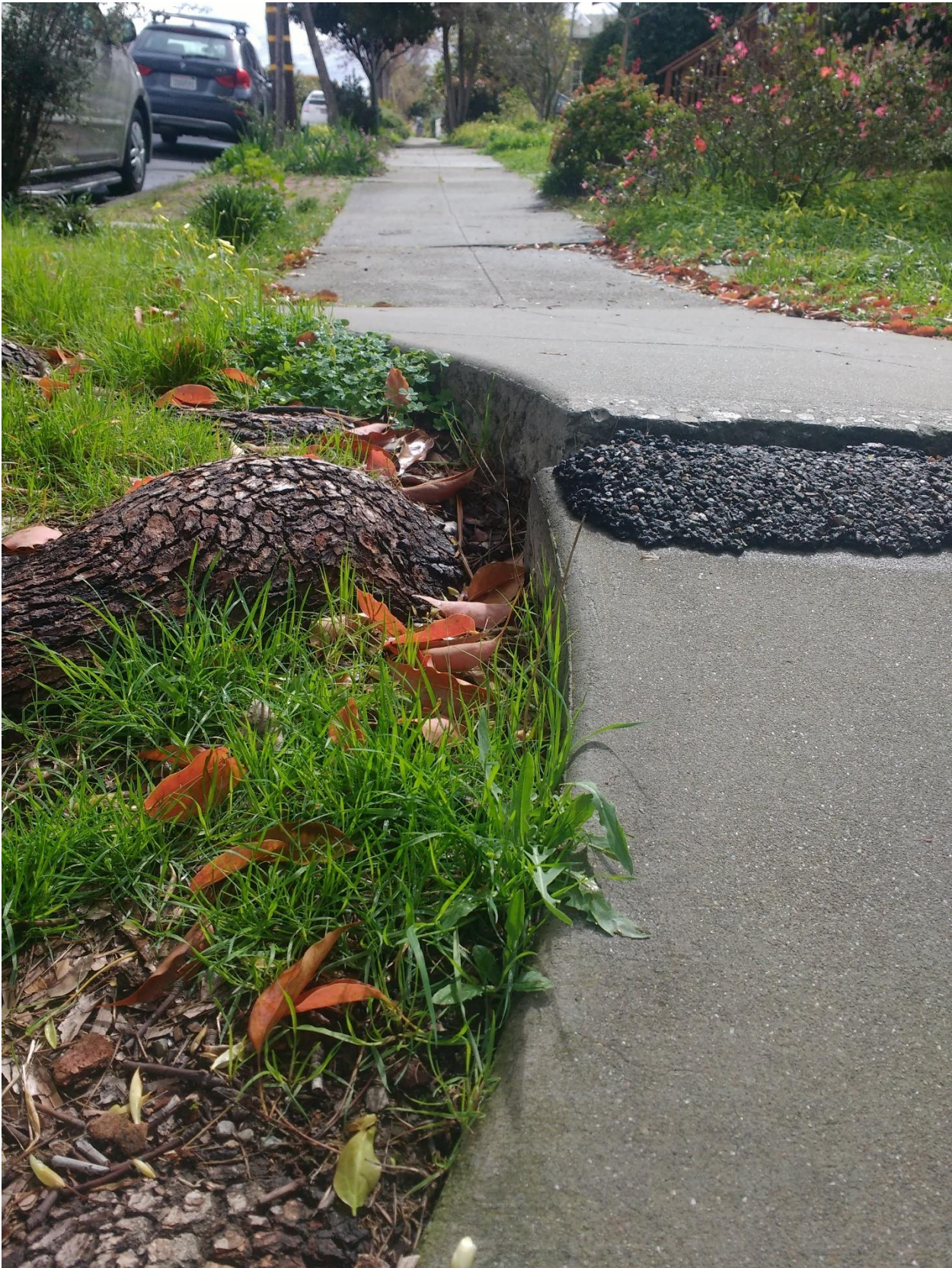
Lifted sidewalk (previously repaired and curved out)
