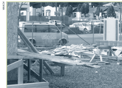
Using a cut-pile such as this one at the Habitat for Humanity Fruitvale development will greatly reduce waste during construction.
