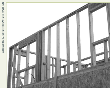
Advanced framing design elements, such as 24-inch stud spacing and headers made from engineered lumber, save resources while improving building performance. This photo was taken during construction at the Fruitvale Habitat for Humanity project in Oakland.
