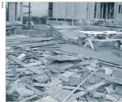
Ends and cut-pieces of joists, siding, framing and other building materials are stockpiled for reuse on this jobsite. Pieces not used are donated or recycled once construction is complete.
