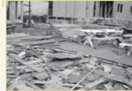
Ends and cut-pieces of joists, siding, framing and other building materials are stockpiled for reuse on this jobsite. Pieces not used are donated or recycled once construction is complete.
