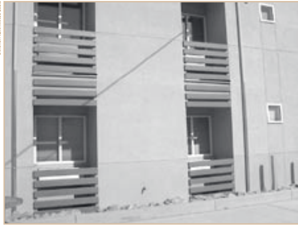
Plastic composite lumber made from recycled plastic and wood pulp functions as trim detail at the El Paseo Studios development in San Jose.
