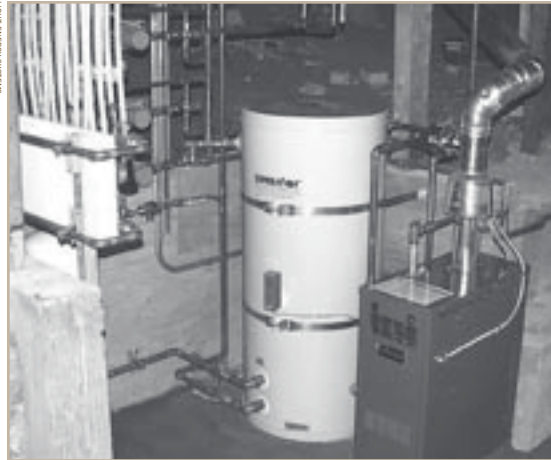
A high-efficiency boiler and storage tank provide hot water for residents and feed a radiant hydronic heating system (white tubing at left).
