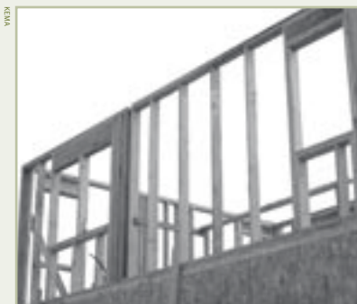
Advanced framing design elements, such as 24-inch stud spacing and headers made from engineered lumber, save resources while improving building performance. This photo was taken during construction at the Fruitvale Habitat for Humanity project in Oakland.
