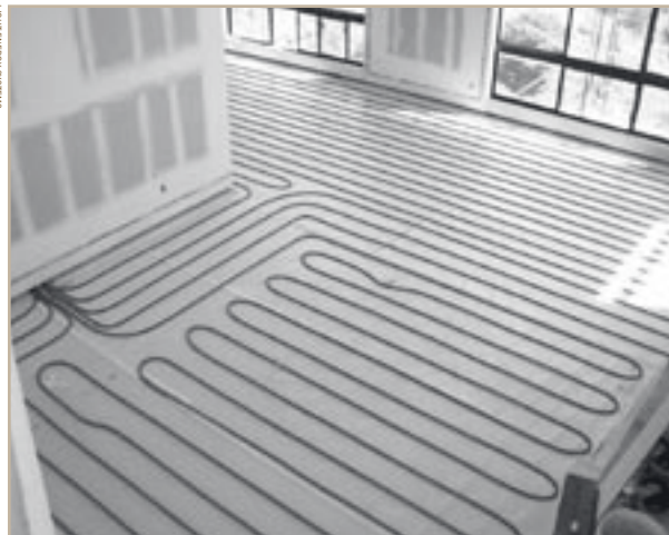
Radiant heating PEX tubing is installed prior to lightweight concrete being poured in this suspended floor application.
