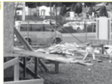
Using a pile such as this one at the Habitat for Humanity Fruitvale development will greatly reduce waste during construction.
