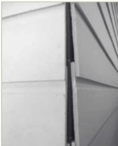
Fiber-cement siding being installed at the Fruitvale Habitat for Humanity project in Oakland.
