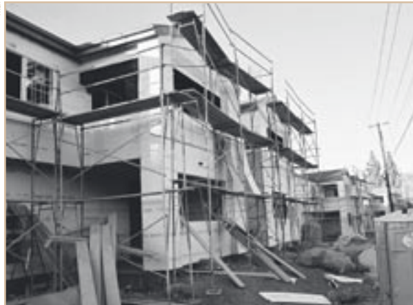
This job site was not vandalized, but it looks as though it could have been. A clean and well-maintained site and building discourages vandals.
