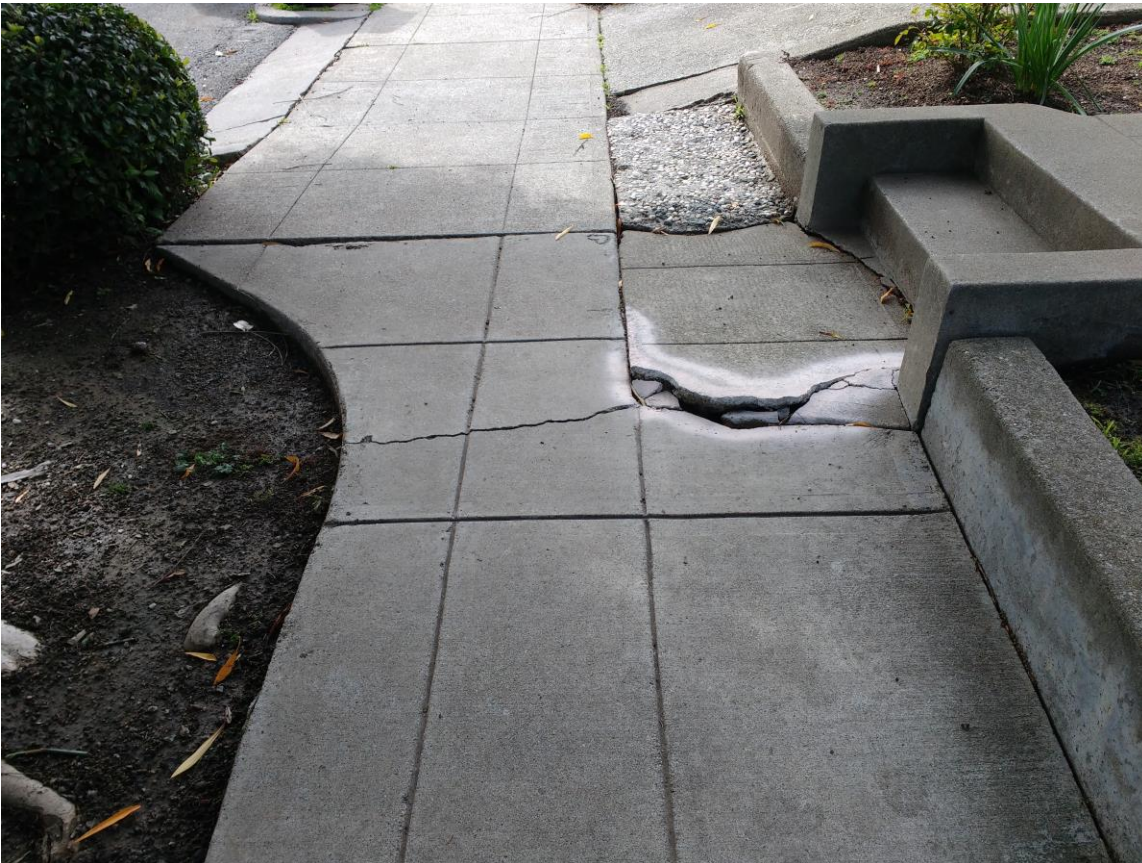
damage to sidewalk
