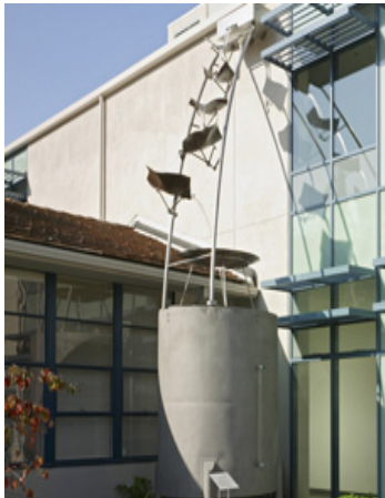
Rainwater is harvested and used to flush toilets in Oakland.
