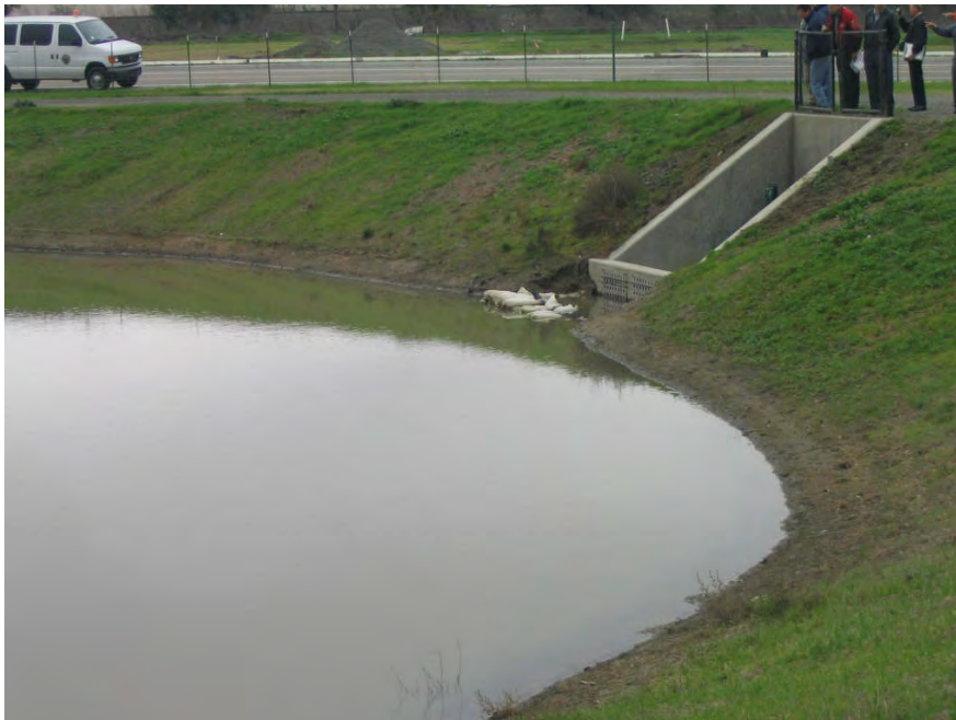
Figure 5-6: Detention pond in Pleasanton provides stormwater treatment and HM.
