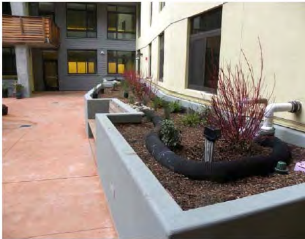
Figure 6-12: Half-buried, perforated flexible pipe serves as a flow spreader to distribute stormwater evenly throughout long, linear flow-through planter in Emeryville (Source: GreenGrid/ Weston Solutions).
