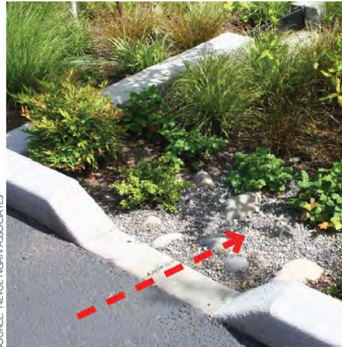
Figure 5-8: This standard curb cut at parking lot rain garden has 45 degree chamfered sides.
