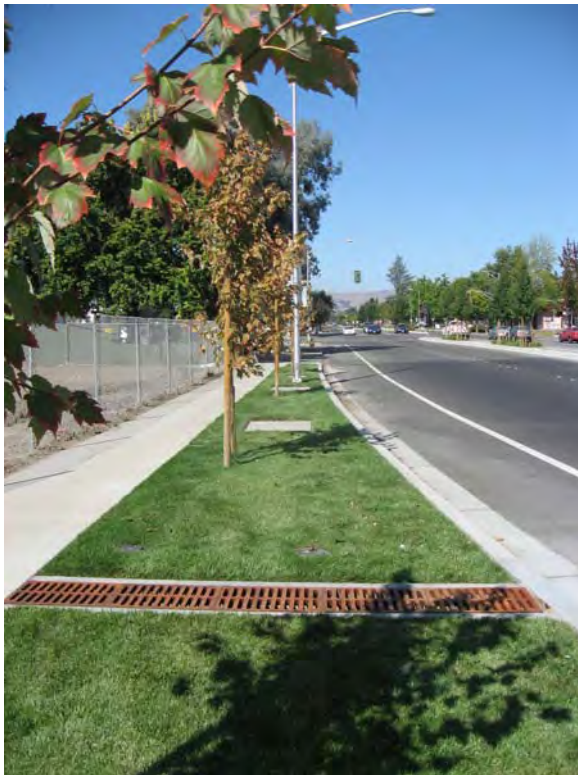
Figure 8-3: Series of non-proprietary tree well filters installed along roadway, City of Fremont
