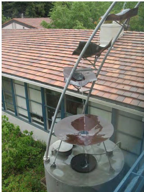
Figure 8-9: Rainwater harvesting system, Mills College, Oakland
