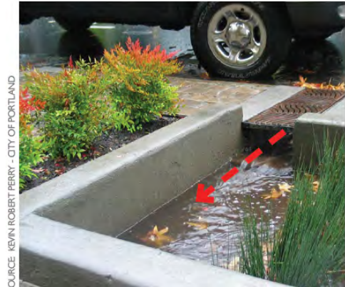
Figure 5-17: A grated curb cut allows stormwater to pass under a pedestrian egress zone to the stormwater facility.
