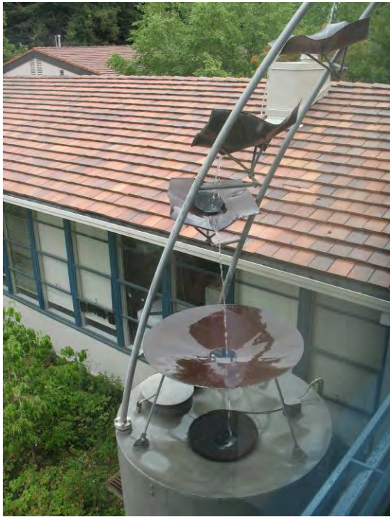
Figure 6-36: Rainwater is collected and used for flushing toilets at Mills College, Oakland.
