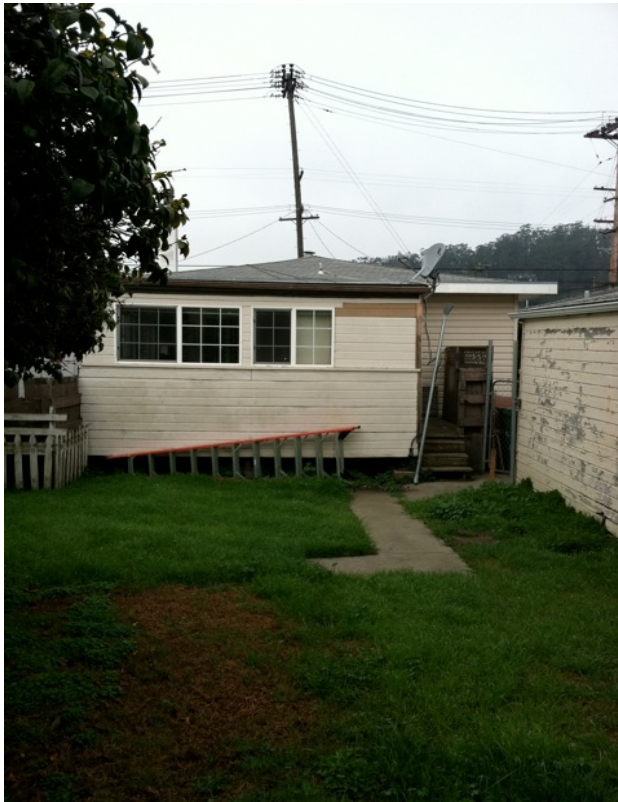
Photo 1. Illegal Rear Addition
