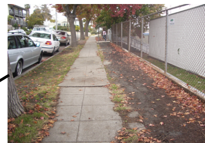
Replace and widen sidewalk along Curtis St. to comply with ADA requirements
