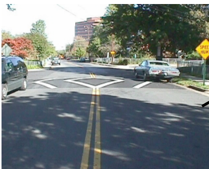
install a speed hump on the 1000 block of Santa Fe Avenue
