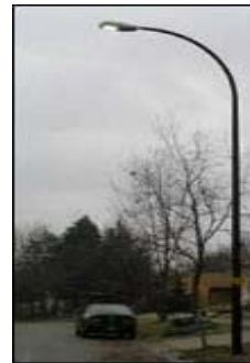
Photo of cobra head street light
